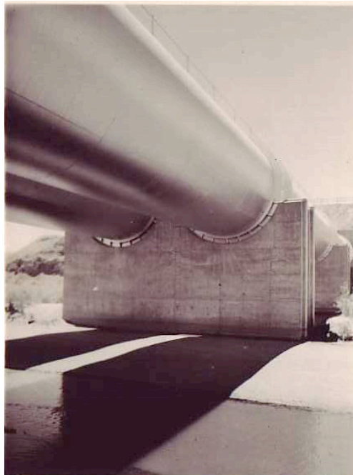
FIGURE 29: All-American Canal (Siphon Across New River) PWA funded, built by Bureau of Reclamation
